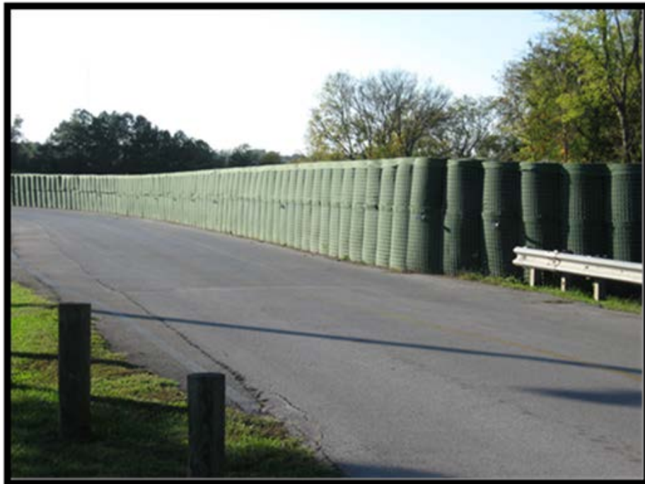
Figure 6: HESCO Bastion Barriers (Photo by Author)
